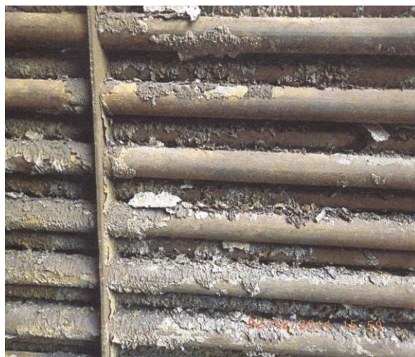
Figura 2 - Middle part of low-temperature section
